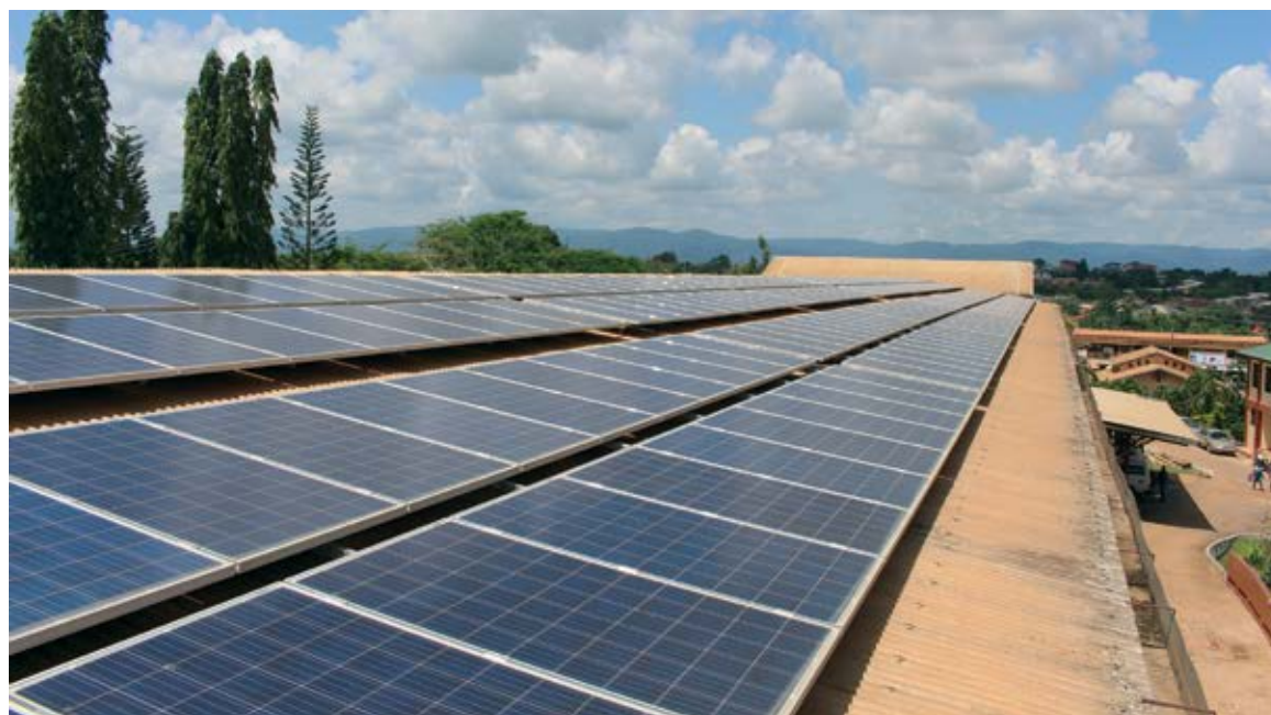
Solar modules at St. Dominic Catholic Hospital in Akwatia in the south of Ghana.
